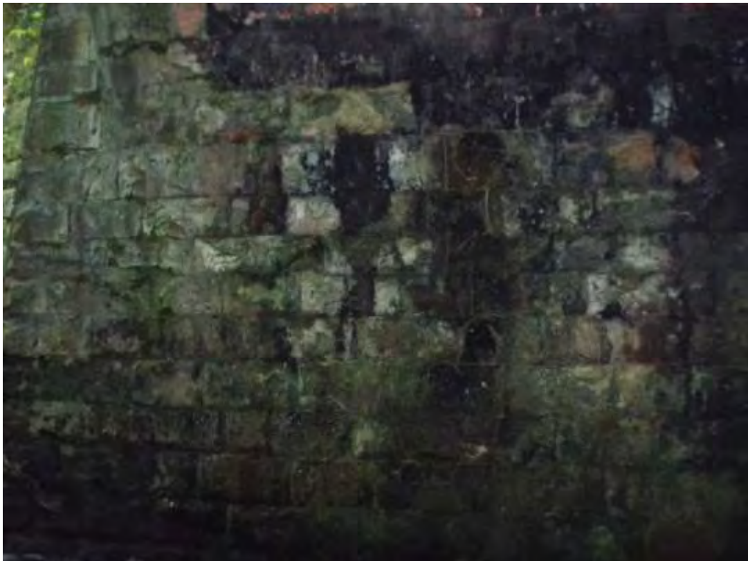
Photograph 16 (P11) - Salt and damp staining (east abutment, north end)
