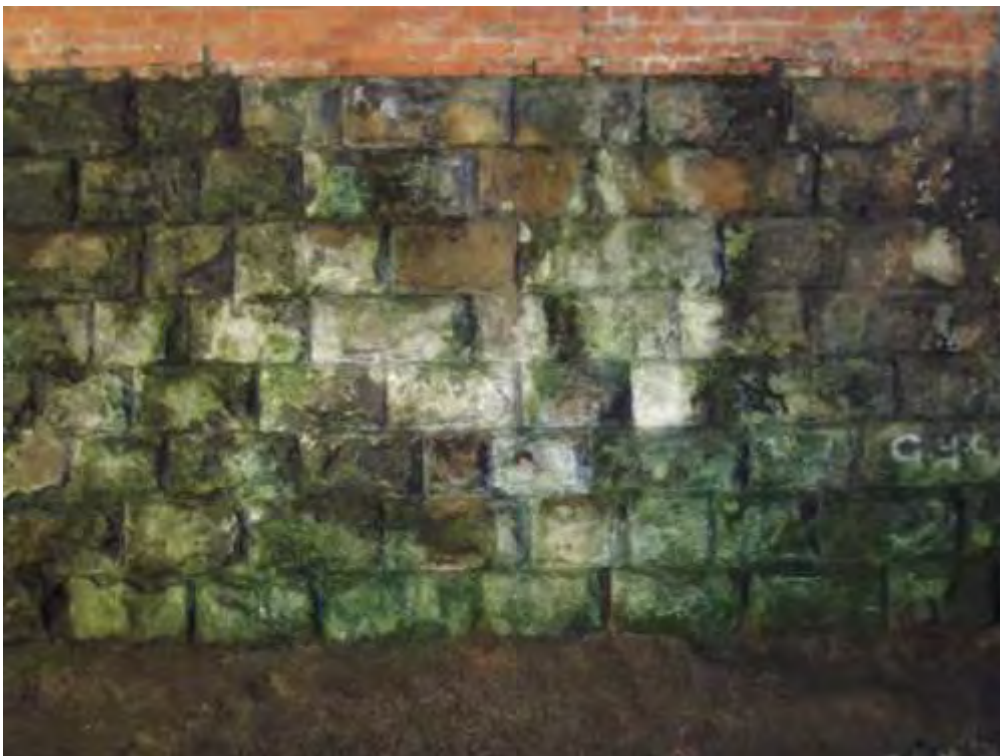
Photograph 14 (P7) - Salt and damp staining (west abutment centre)
