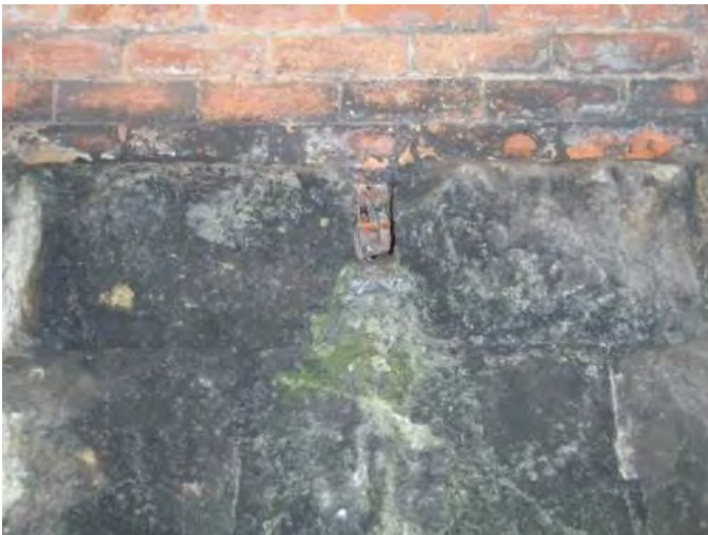
Photograph 20 (P9) - Gap in stonework (west abutment)
