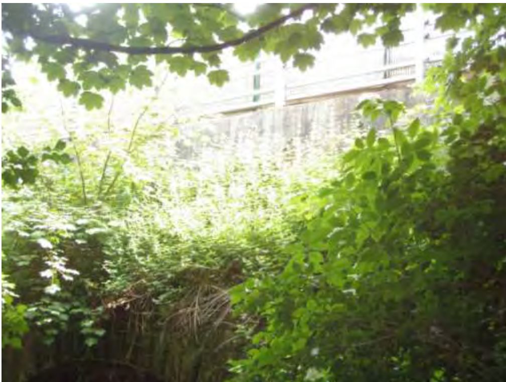
Photograph 26 (P31) - Vegetation covering carriageway retaining walls
