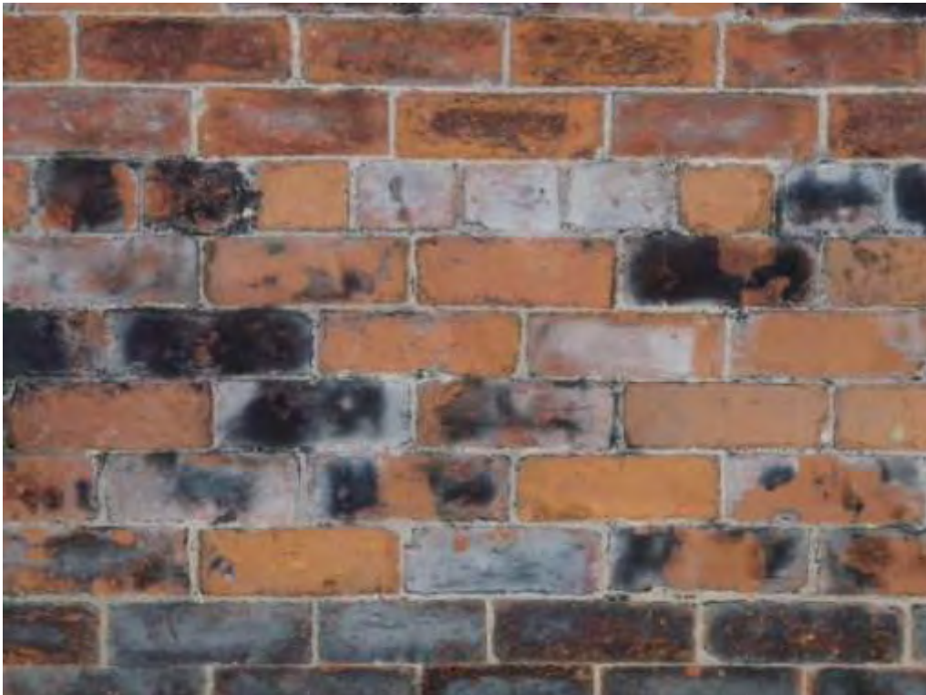
Photograph 12 (P17) - Spalling of brickwork surface and salt staining (soffit)
