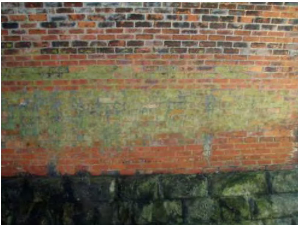
Photograph 10 (P16) - Algal staining to soffit (east abutment side)
