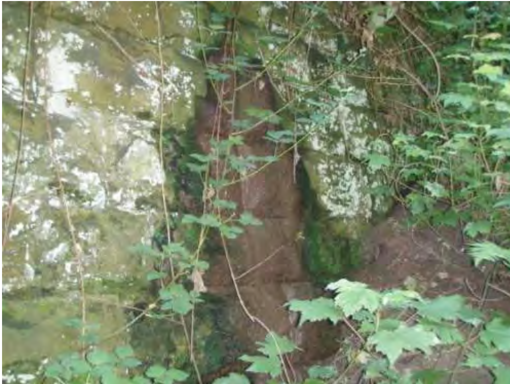
Photograph 23 (P24) - Damp (north west wing wall)
