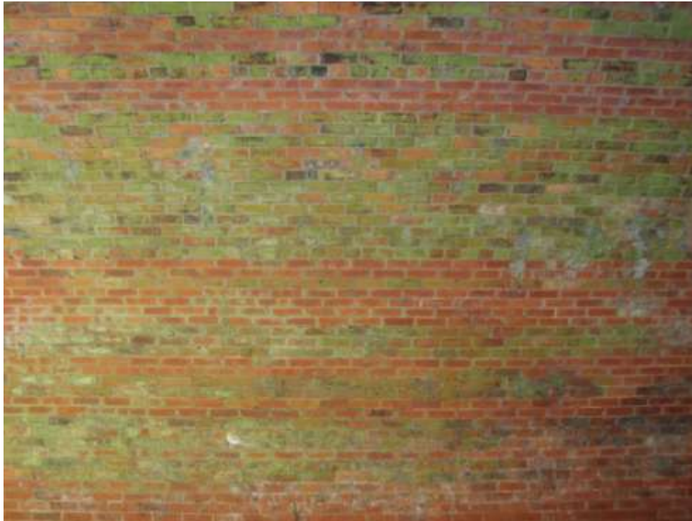
Photograph 9 (P15) - Algal staining to soffit
