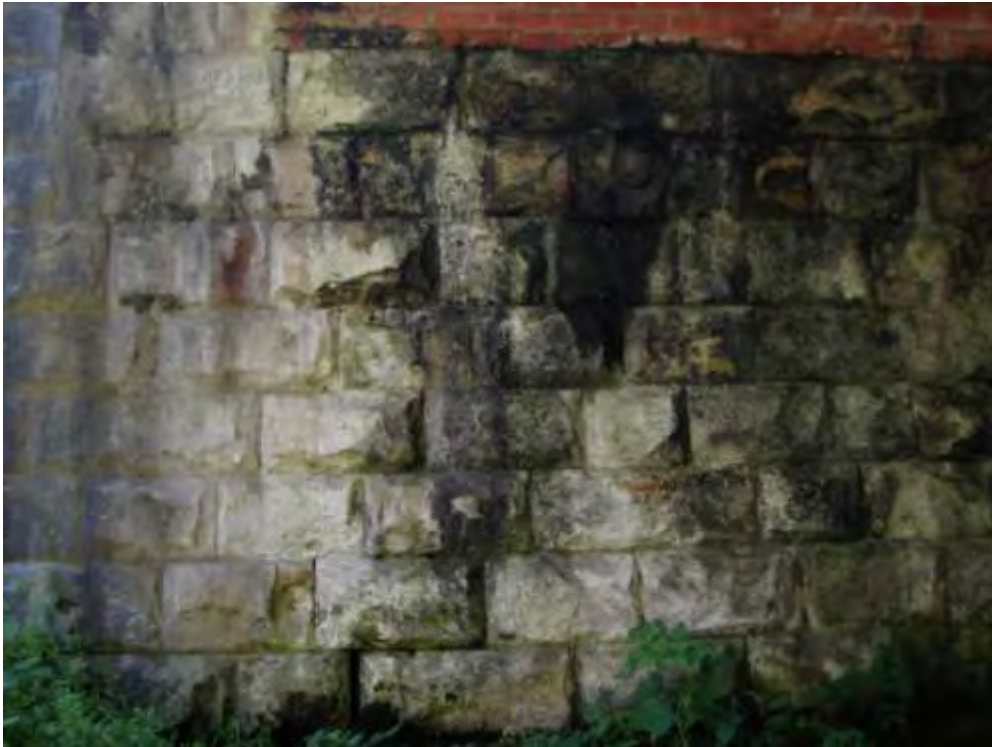
Photograph 13 (P6) - Salt and damp staining (west abutment, south end)
