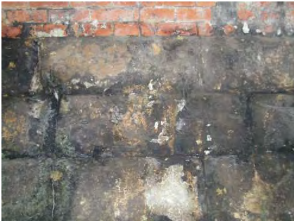
Photograph 18 (P8) - Spalling stonework surface (centre of west abutment)
