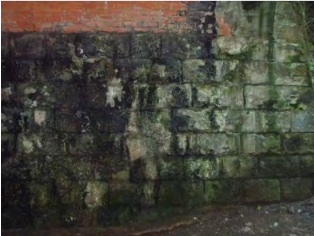
Photograph 15 (P10) - Salt and damp staining (west abutment, north end)
