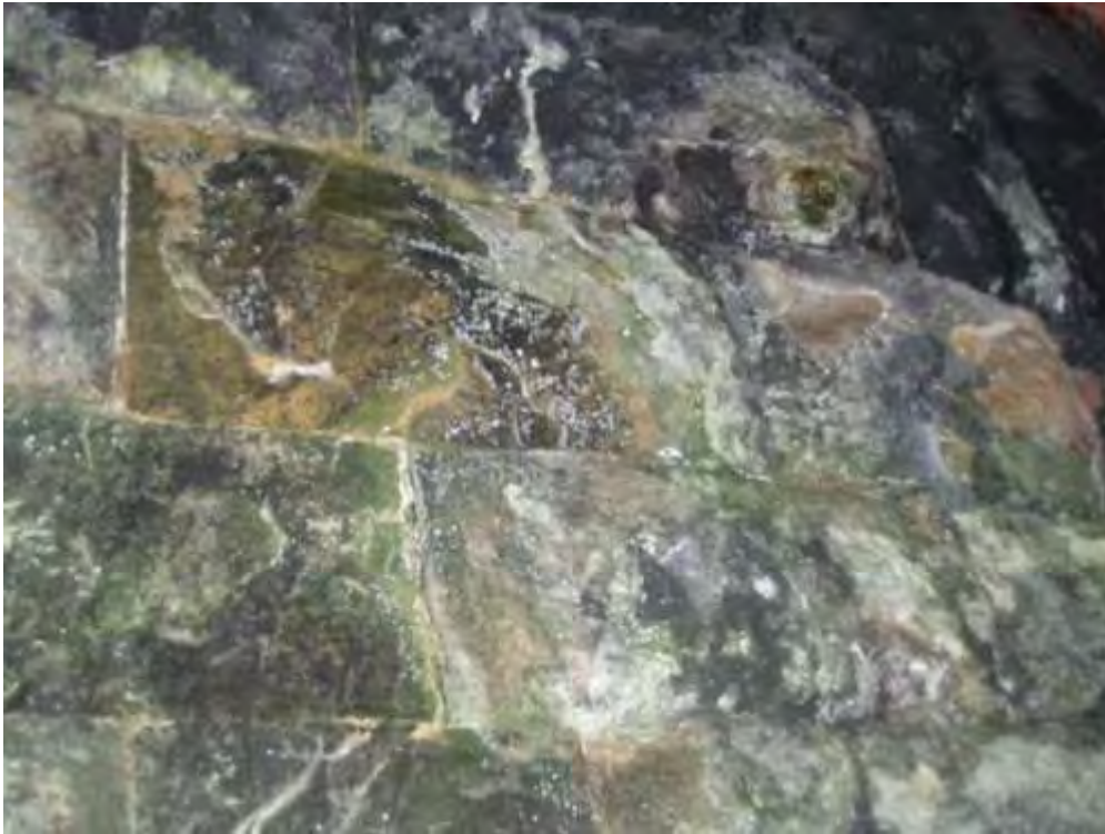
Photograph 19 (P12) - Spalling stonework surface (east abutment)
