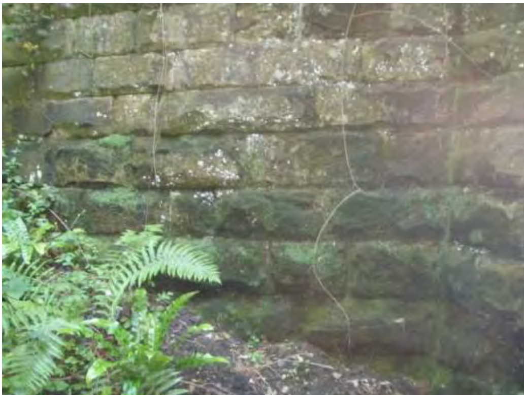
Photograph 22 (P23) - Damp and lichen growth (north east wing wall)
