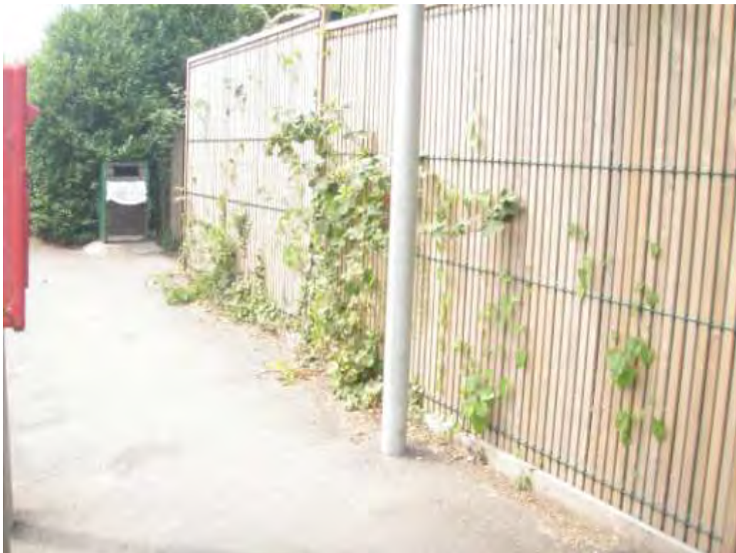
Photograph 28 (P30) - Vegetation coming through wooden fence (north fence)
