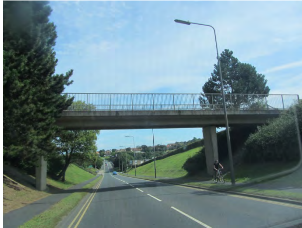
Photograph 23. Airy Hill Footbridge on A171 looking south shows signs of previous bridge strikes.
