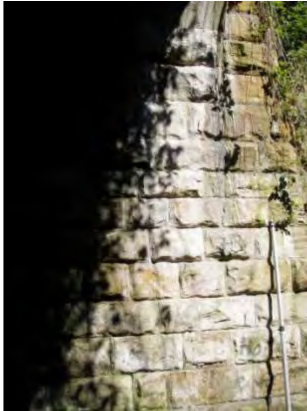
Photograph 17 (P14) - Salt staining (east abutment, south end)
