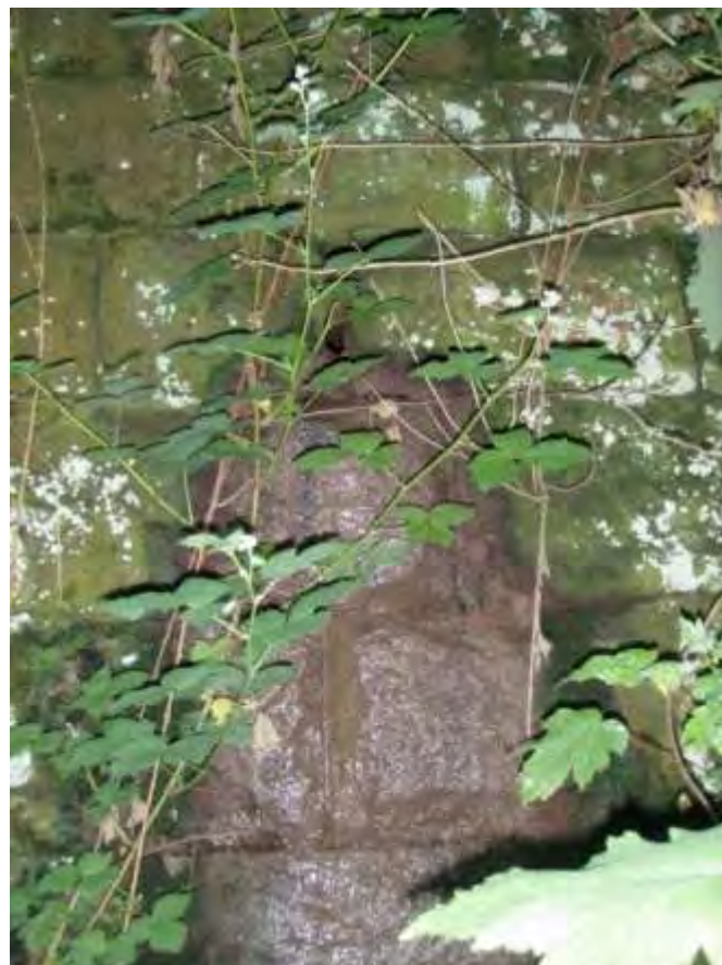
Photograph 24 (P25) - Gap in stonework and damp emanating (north west wing wall)
