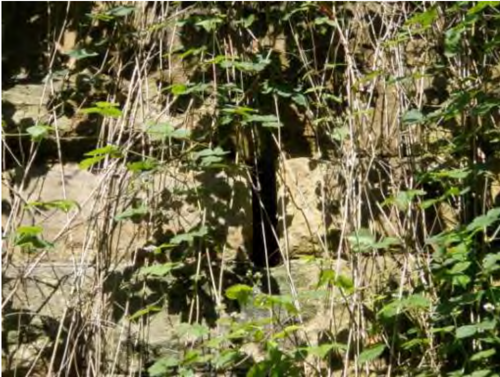
Photograph 25 (P5) - Gap in stonework (south east wing wall)
