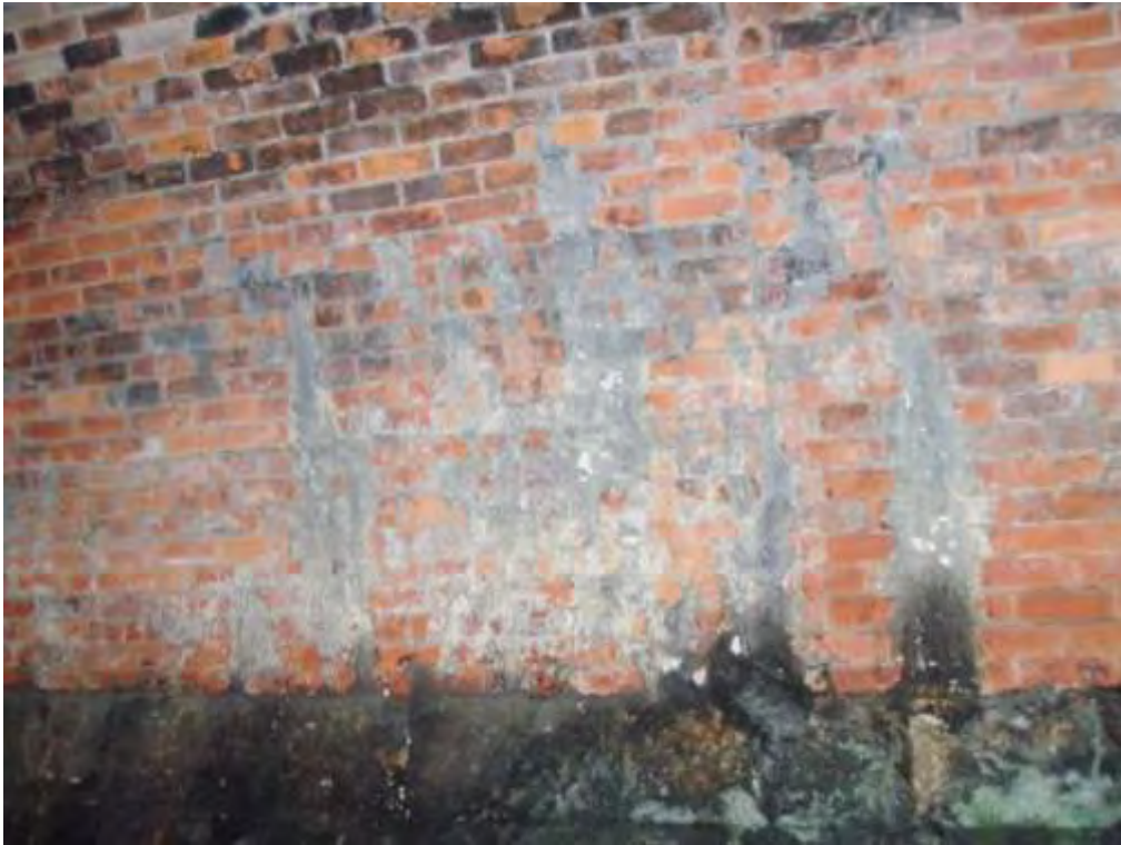
Photograph 11 (P18) - Efflorescence to soffit (east abutment side)
